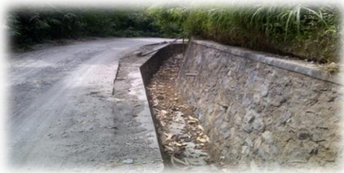
Drainage and retaining wall in Jarakah Village
